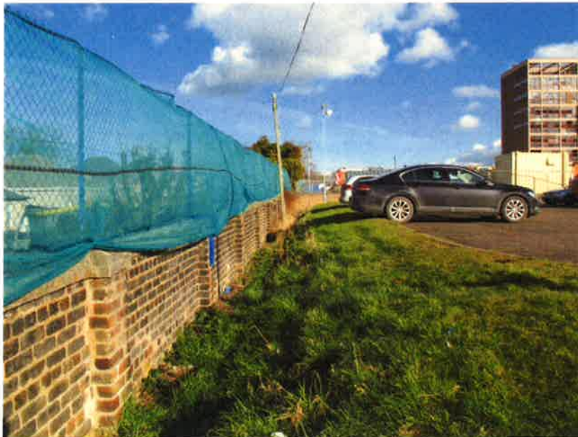
Photo 1 - Existing north boundary. Photo 1 illustrates the existing situation to the north boundary whereby the ground levels were artificially raised to form a level car parking area.
